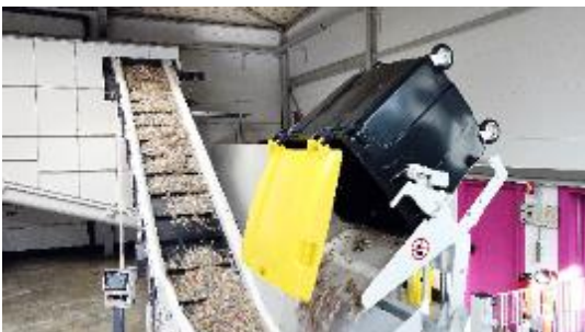
Photo 2: Material that has been pre-shredded and freed of ferrous metals is moved from containers to the conveyor system.
